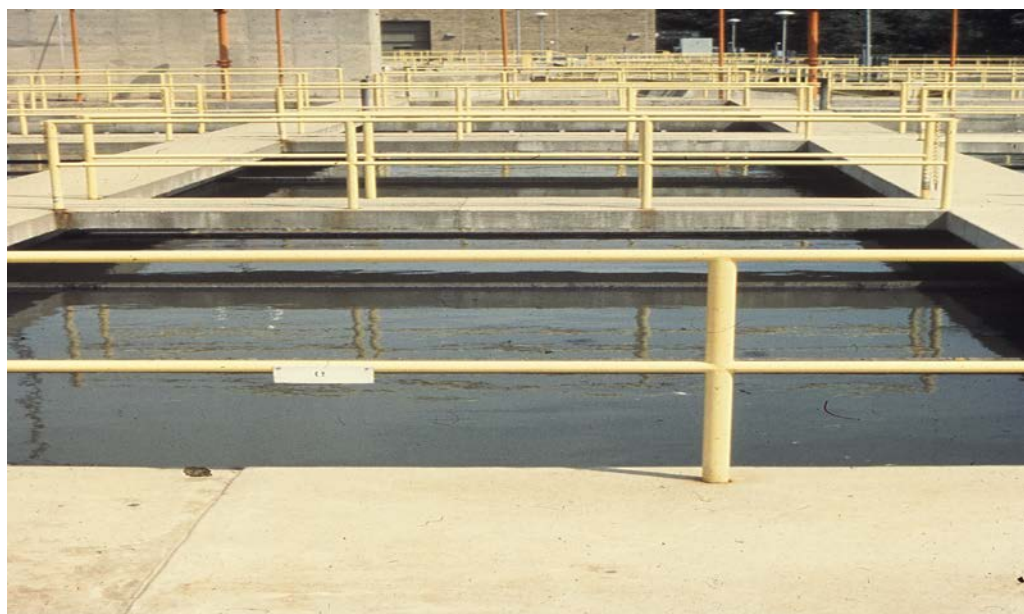
Primary settling tank
