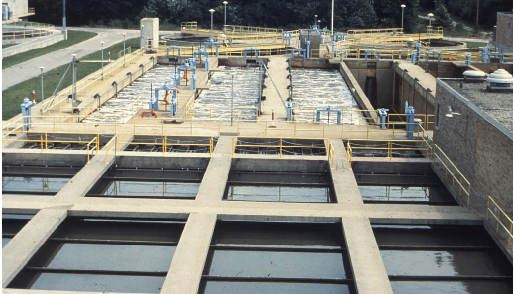
Primary settling tanks in foreground followed by aeration tanks and circular secondary settling tanks
