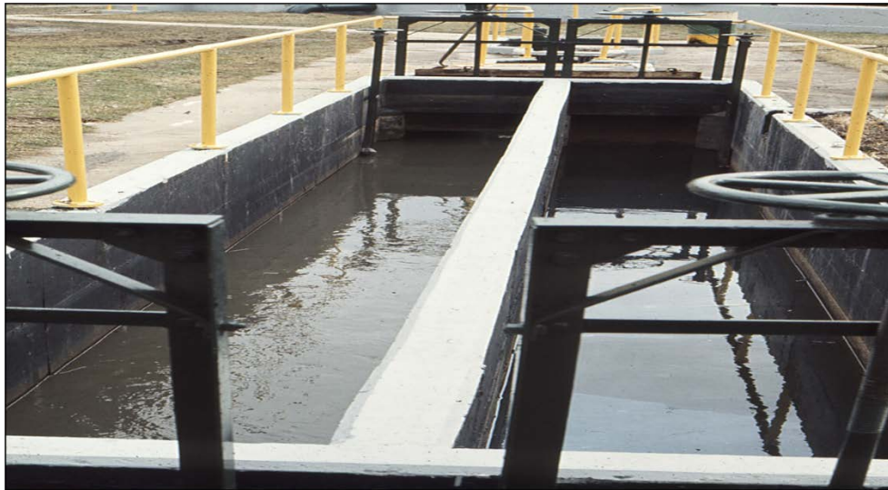
Velocity Controlled Grit Chamber. Left Chamber in Service. Right Chamber Out of Service.
