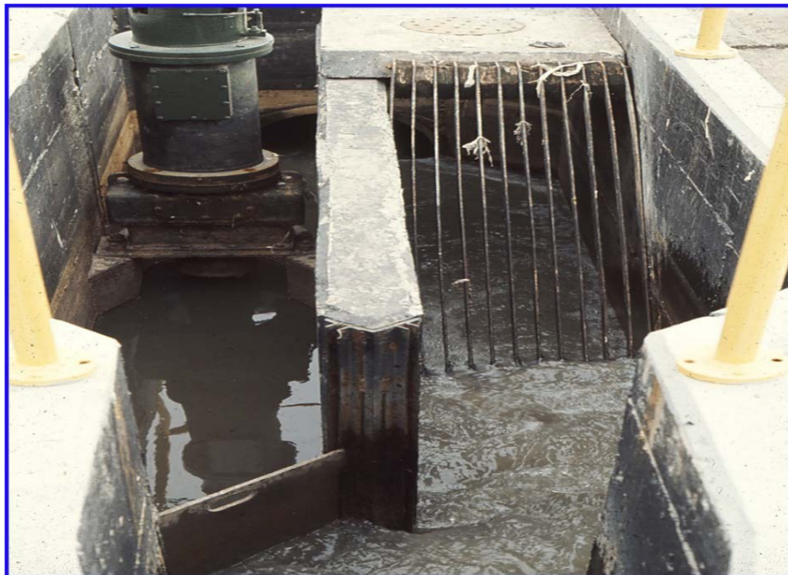
Bar rack (right) and comminutor (left) in a wastewater Treatment Plant
