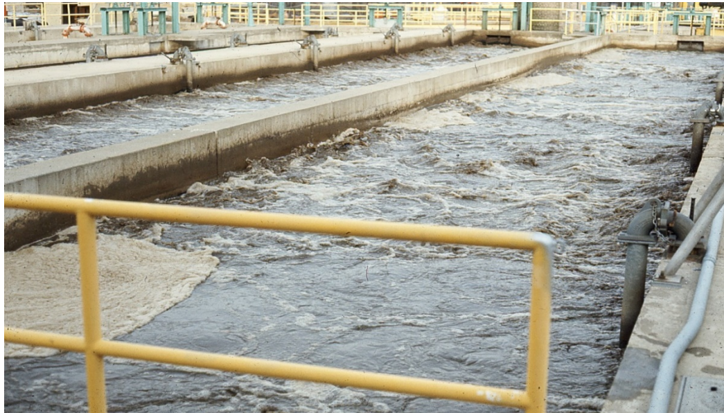
Activated Sludge Aeration Tank
