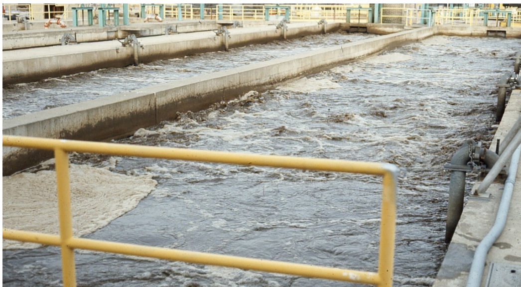
Activated Sludge Aeration Tank
