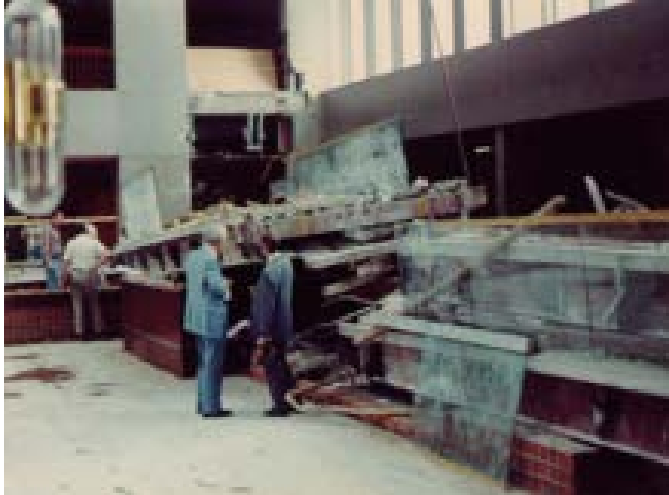
General view of the lobby floor, during the first day of the investigation.
