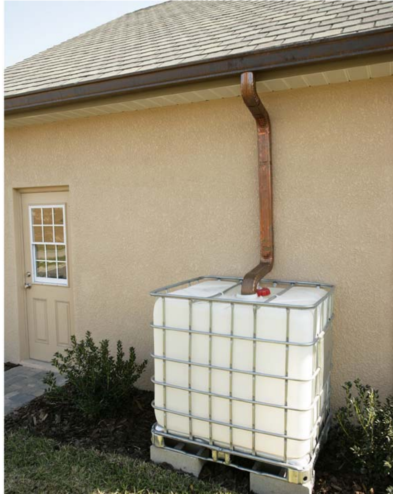
Rooftop collection system
