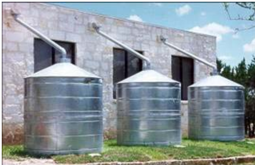
Functional Cisterns– not pretty but also not yet camouflaged
