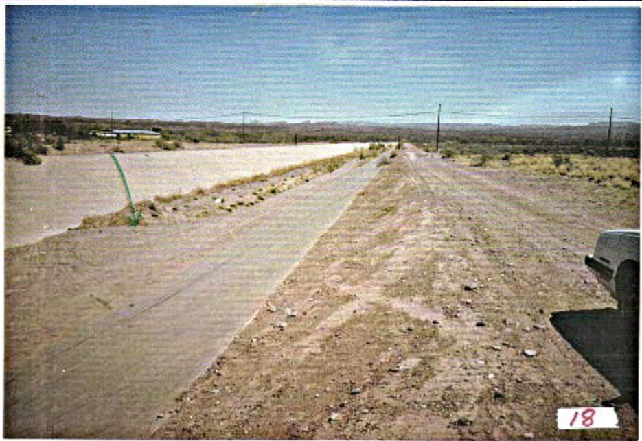
Photo 4. Headcutting induced by pilot channel
