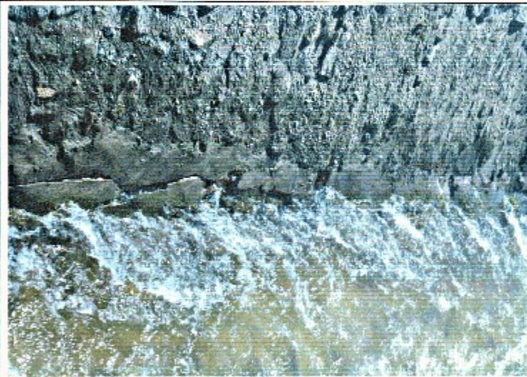
Photo C-14. Spalling at Waterline, 1998
