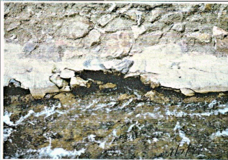
Photo C-13. Spalling at Waterline, 1994
