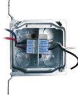
Emergency Relay Figure 6
