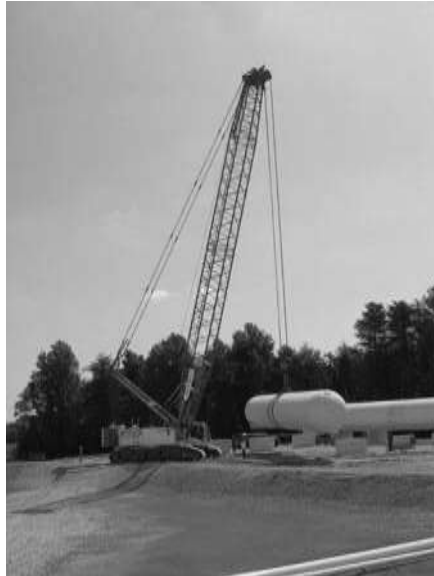
Figure 1.1. A crawler crane can rent for as much as $10,000 per week.
